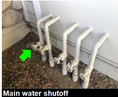
Main water shutoff
