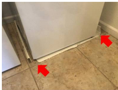
Damaged drain pan
