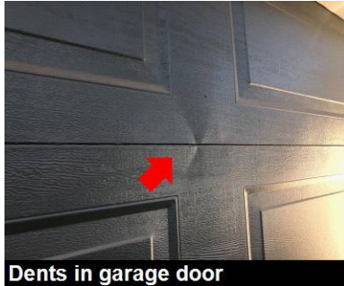
Dents in garage door
