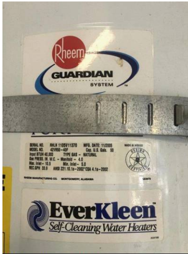
Water heater ID tag
