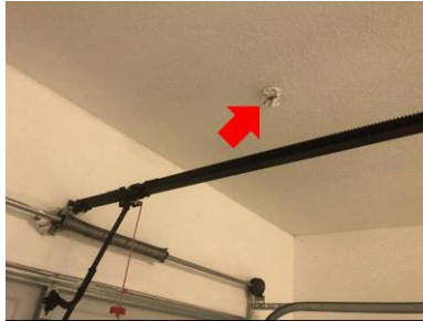
Sprinkler heads are taped up
