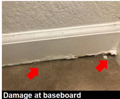
Damage at baseboard
